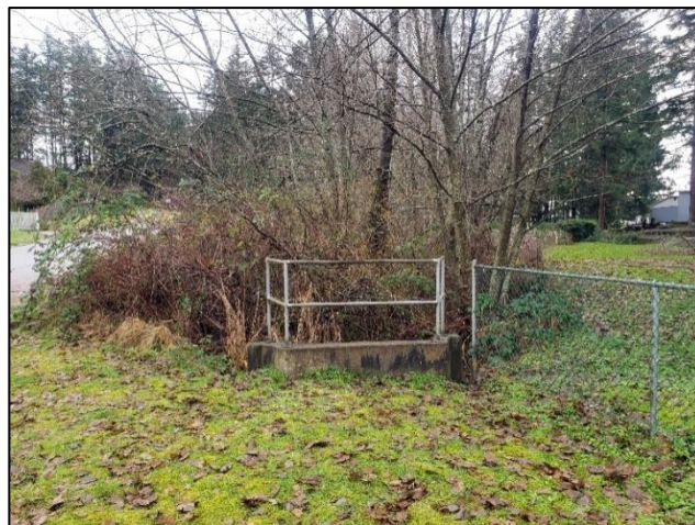
Photo 4. Southeast (downstream) view of the storm sewer outlet headwall at the northwest property corner.
